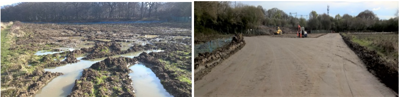
Silty plastic clays with high water table at Shenfield Network Rail before and after RoadCem stabilisation
