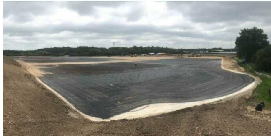
48 hours after the in-situ soils have been stabilised a thin bonding course is applied
