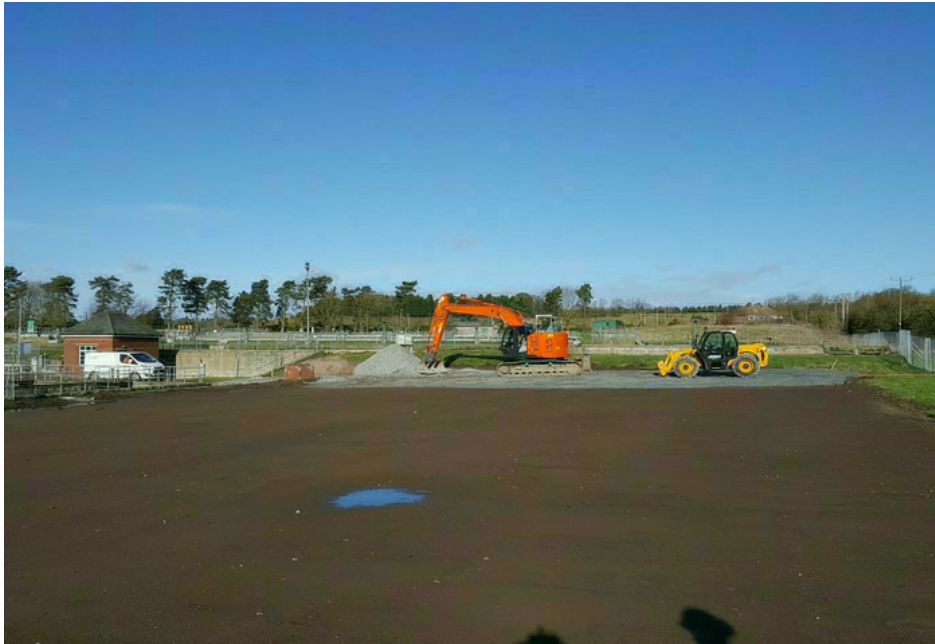
An impermeable operating slab for the washing of bio filter media.
