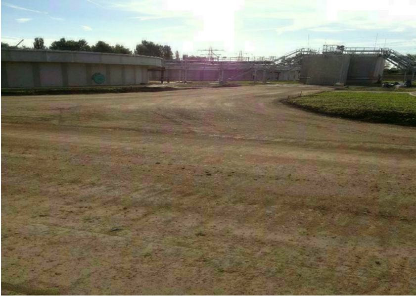
Un surfaced RoadCem bound soil base photographed after two years construction plant trafficking.
