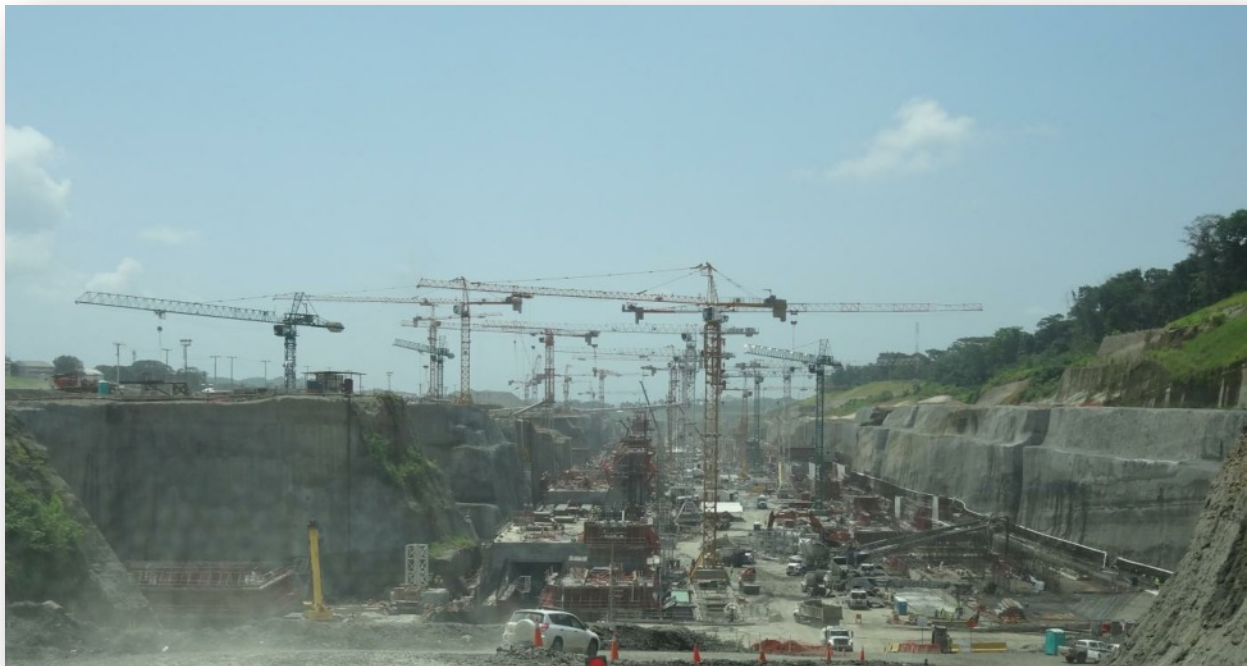
Figure 1: Impression of the construction works on the locks at the Atlantic Site, June 2012
