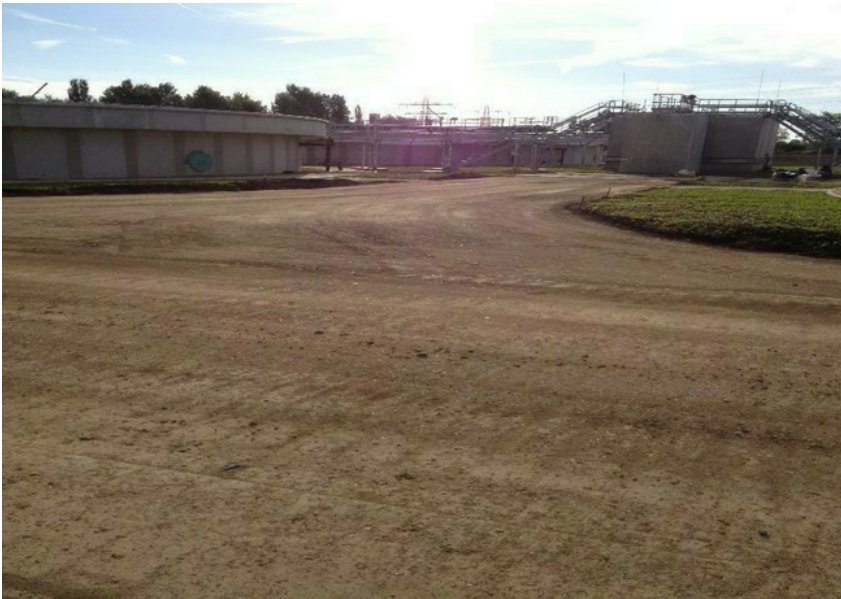
RoadCem soil concrete base photographed after two years construction plant trafficking.
